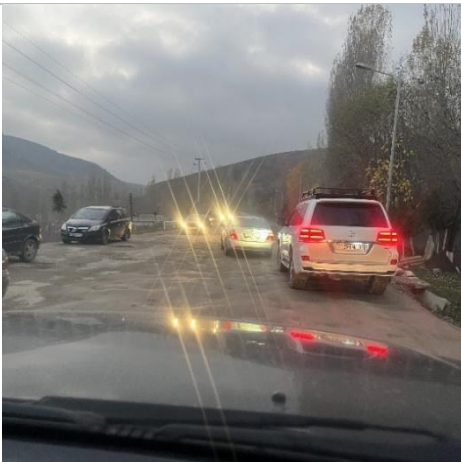
Photo 3: Congested traffic on a pothole-ridden road underscores the urgency of repairs and better traffic flow management.
