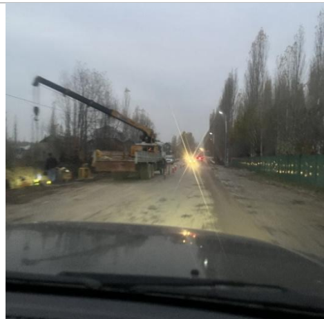
Photo 4: Roadside construction with limited lighting and uneven surfaces highlights the need for traffic control.
